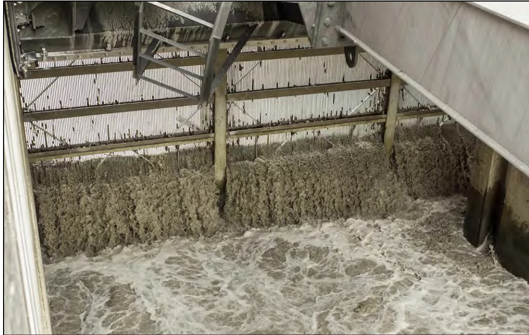
Figure 21: Headloss across trash rack due to clogging by debris.
